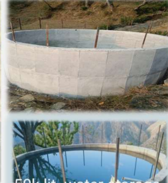
50k lit. water storage tank at Jarwa cluster
